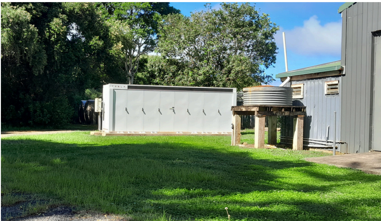
Image: Tesla battery at Powerhouse
