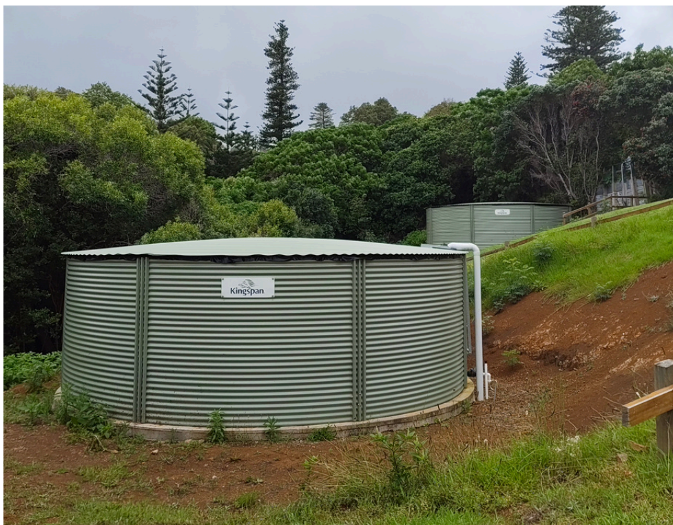
Image: Water tanks at TR Units
