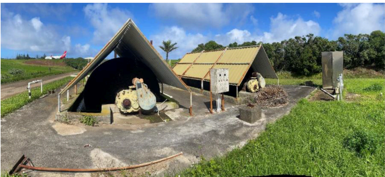
Image: Rotating Biological Contactors (RBC) - Wastewater treatment plant
